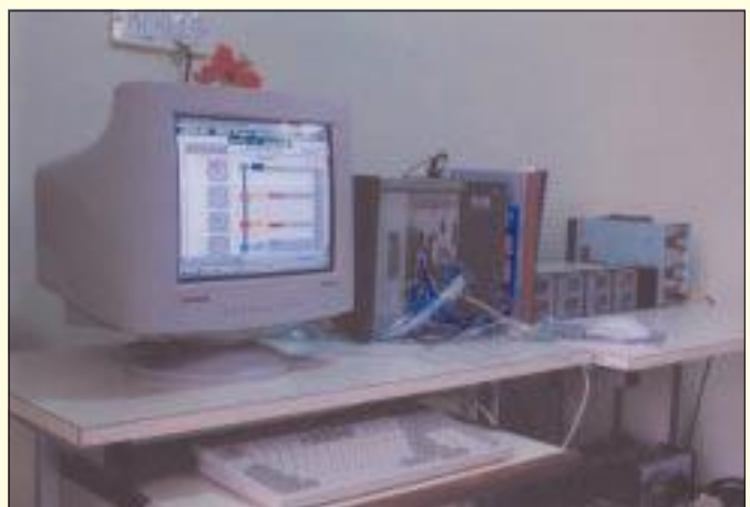
Data Logger for the SRI Meteorological Tower at Anupuram Township, Kalpakkam
