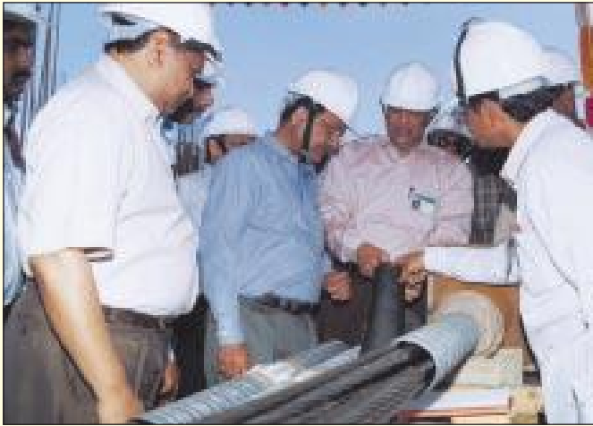
Chairman, AERB (Second from left) and Shri. V.K.Sharma Senior Executive Director, NPCIL examining a Sample of the Stressing Cable
