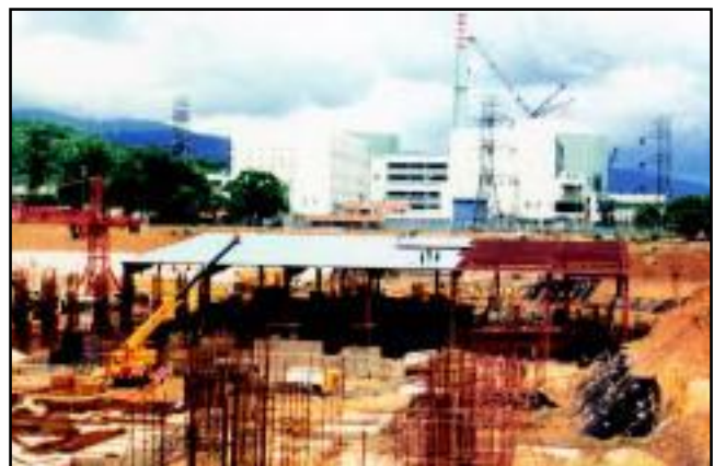
Kaiga Atomic Power Project Units - 3 & 4
