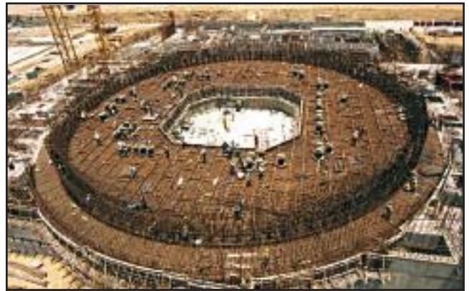
Construction Activities in Progress at + 5.4 m slab of RB of Unit-1 of KK-NPP.
