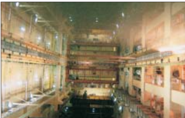
TAPP-3: Filling of SFSB after Major Modification.
