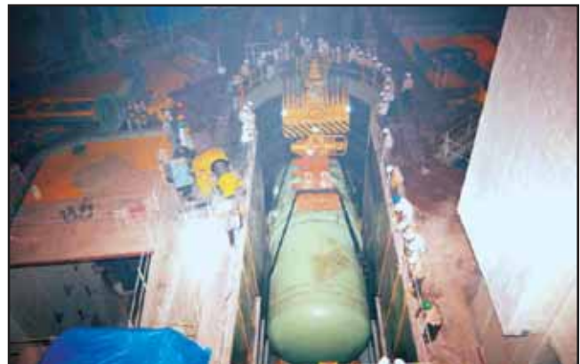
KK-NPP Unit-1: RPV Positioned Horizontally prior to installation in the Reactor Cavity
