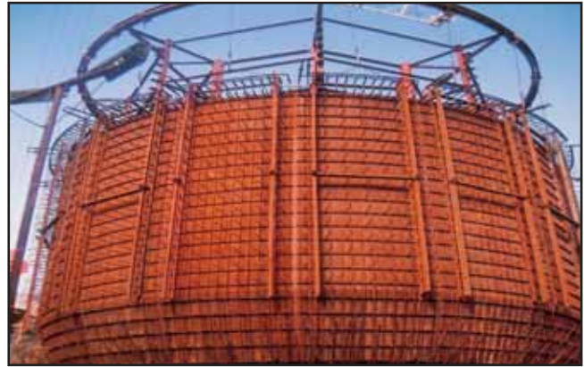
Reactor Vault Liner with Biological Shield Cooling Pipes of PFBR
