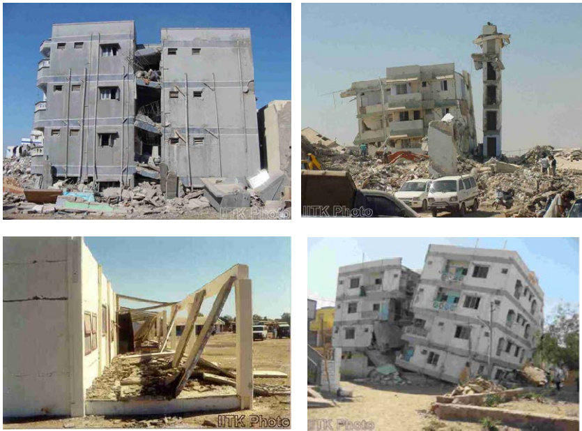
Figure 11 - Structural failures during Bhuj earthquake 2001 [Source: www.nicee.org (W6)]
