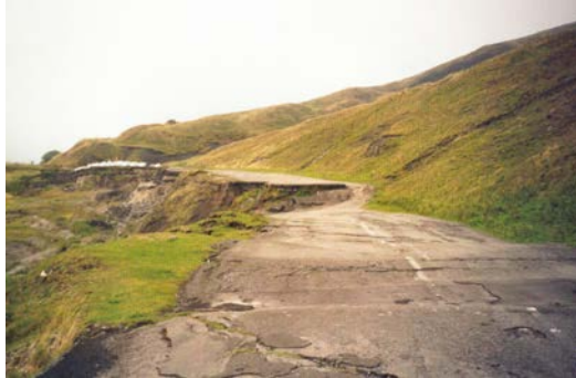
Figure 13 - Subsided road [Source: Wikipedia commons (W5)]
